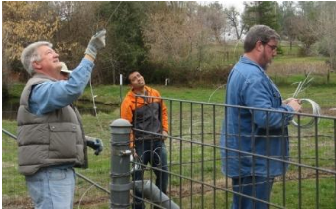
Lonnie KI6ZYY, Augustine KK6ICE and Dan KJ6RGX making sure there were no kinks in the guy wiring.
