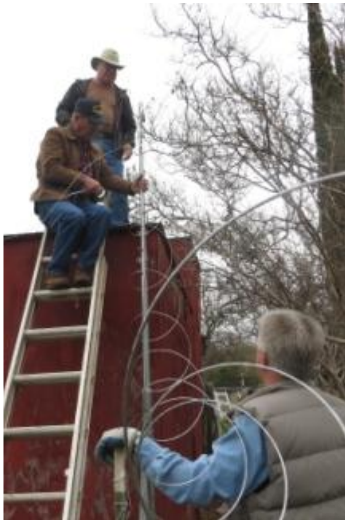
Lonnie KI6ZYY (on the ground), Lee KC6MCI (on the ladder) & Curtis KF6VFP (on the shed roof). We are standing the center mast up and uncoiling the guy wire.
