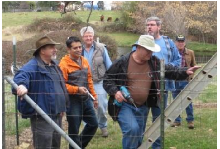
Mike KM6EBY, Augustine KK6ICE, Lonnie KI6ZYY, Dan KJ6RGX and Lee KC6MCI watch as Curtis KF6VFP goes up the ladder.
